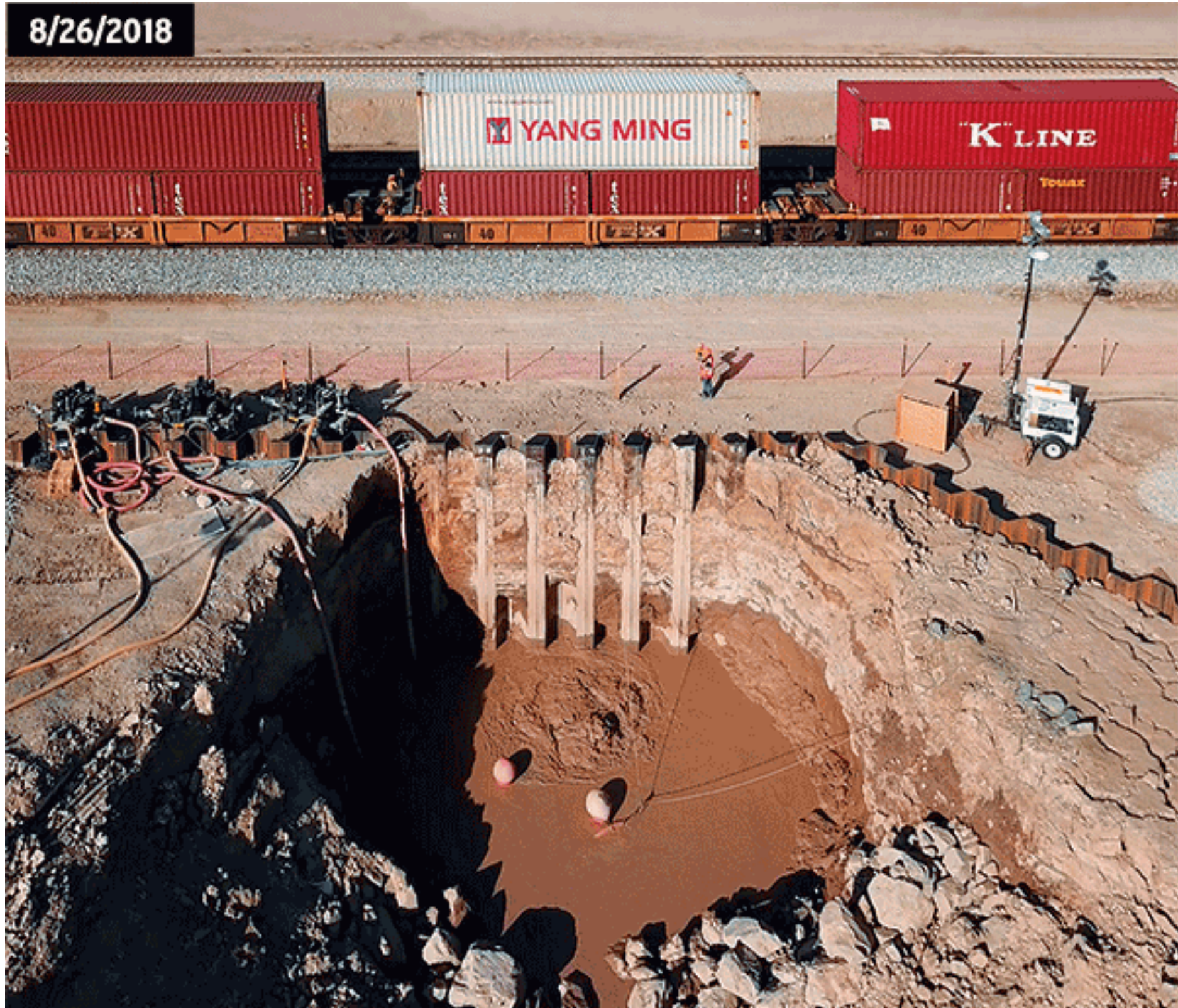
A 140 ft long sheet pile wall was constructed to slow W9a's southwesterly movement. (David K. Lynch)
